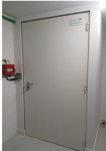
Figure 3: Secured door and connections for the optical fiber and electricity
