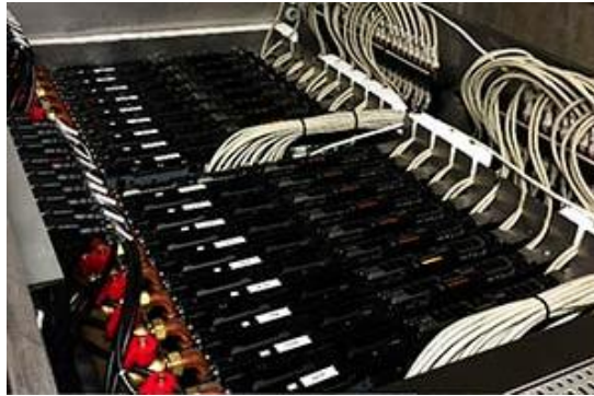
Figure 1: Servers immersed in oil
