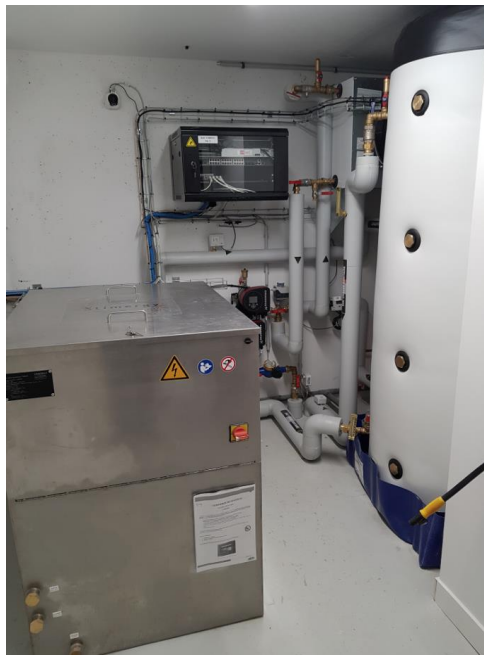
Figure 7: Tebios and water tank in the second boiler room
