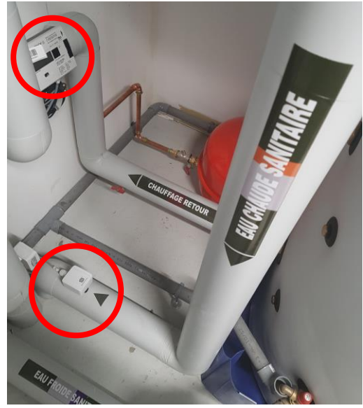
Figure 19: Temperature sensors and calorimeter in “Oiseau des Iles” building
