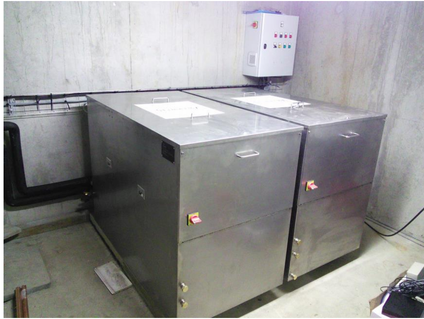
Figure 10: The two boilers
