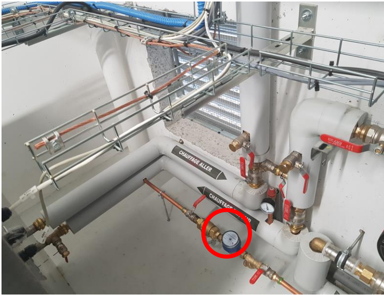
Figure 18: Flowmeter installed in the boiler room in “Oiseau des Iles” building
